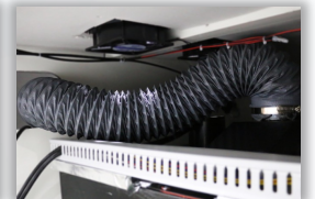
Fume Extraction System
