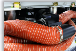
Fume Extraction System
